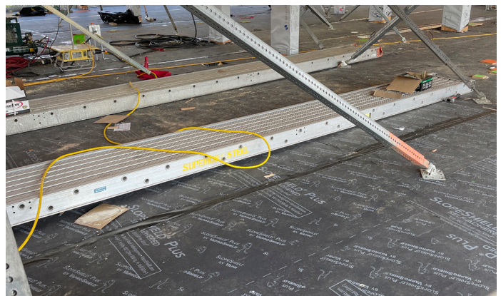
By protecting the interior floors with SlopeShield Plus SA, work can commence on the lower floors helping to keep the project on schedule. Installation: Multi-Family, Seattle, WA
